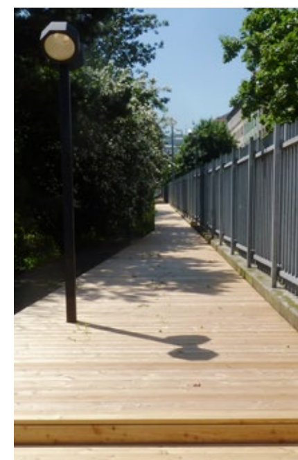
The opening up of the site with the help of a 140m long wooden walkway.
